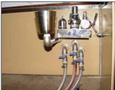
Boiling Pan Double Jacket Water Level Controlling
